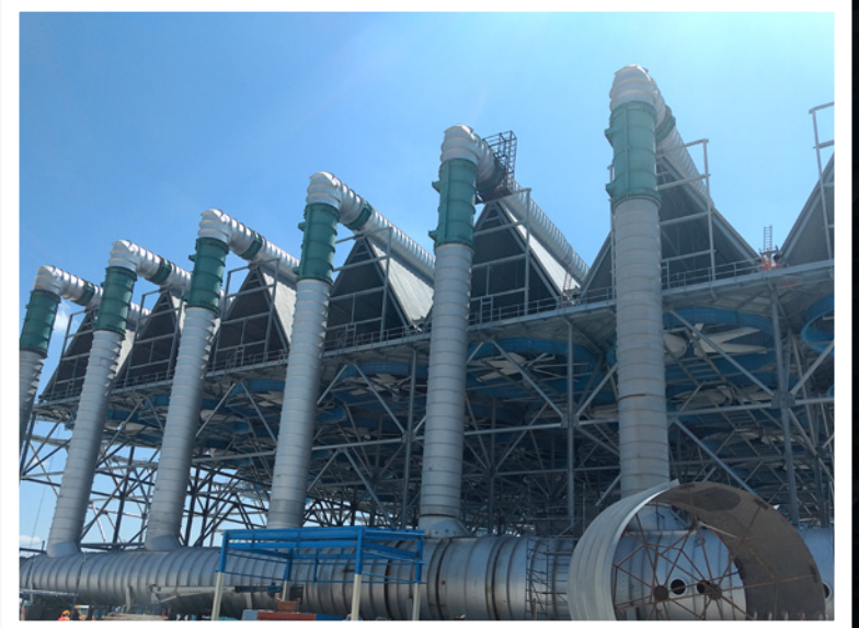
Air-cooled steam condensers
